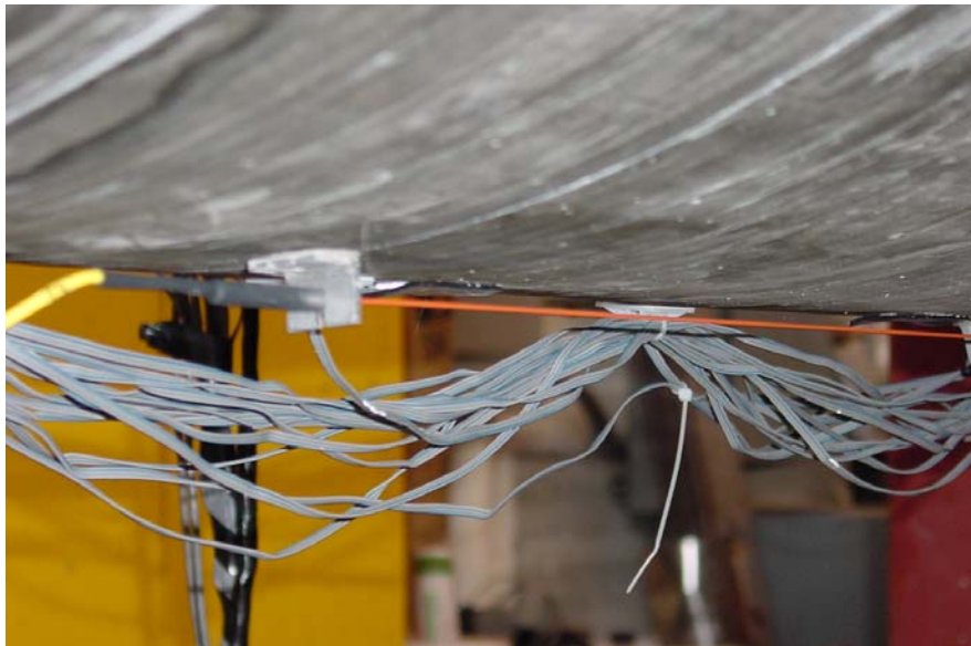
Figure 4. Long-gage fiber grating sensor surface mounted with brackets along bottom edge of girder.
